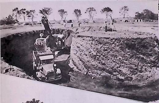
A power shovel does work in short order on site of New York's Perisphere
