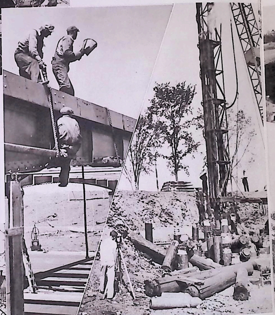
At site of 1939 World's Fair a 100-foot pile driver sinks supports for 700-foot Trylon at rate of twenty a day
