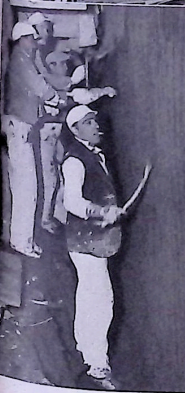
Above: Plasterers at work on the Hall of Mines and Metallurgy. Top: Pouring concrete for the Trylon foundations. In the center of the picture is the circular concrete base of the Perisphere and beyond
